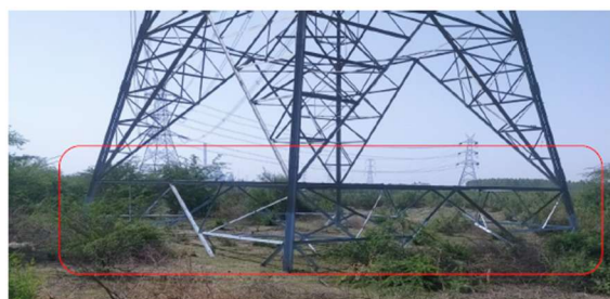
Observation-1- Tower No. 11: Members of tower been theft
