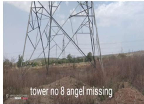
Tower No. 8: Member Missing
