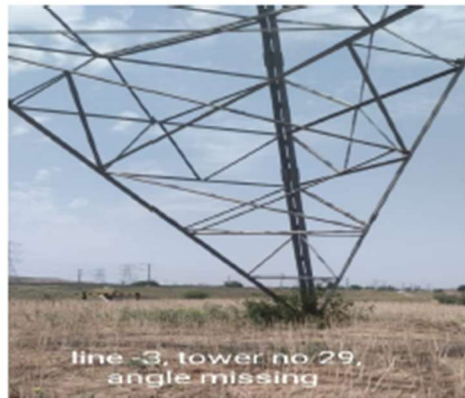
Tower No. 29: Member Missing
