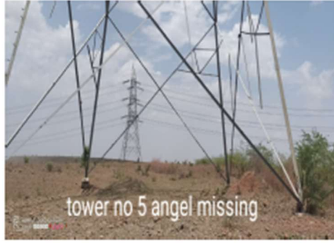
Tower No. 5: Member Missing
