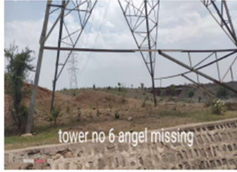
Tower No. 6: Member Missing
