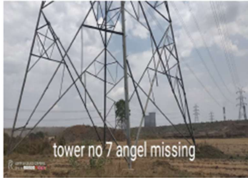
Tower No. 7: Member Missing
